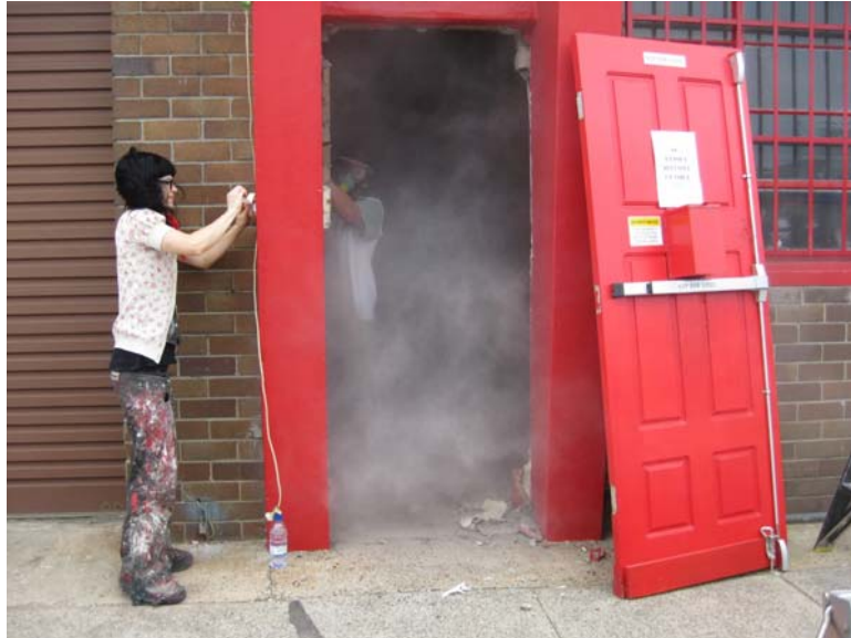
Penelope Benton of the Red Rattler, bringing a doorframe into compliance with conditions required for Council for the issue of a liquor licence. Photo: Penelope Benton
